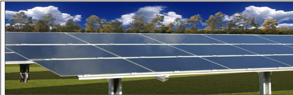
Plate 3-2: Frontal view of PV arrays mounted on fixed mounting systems
