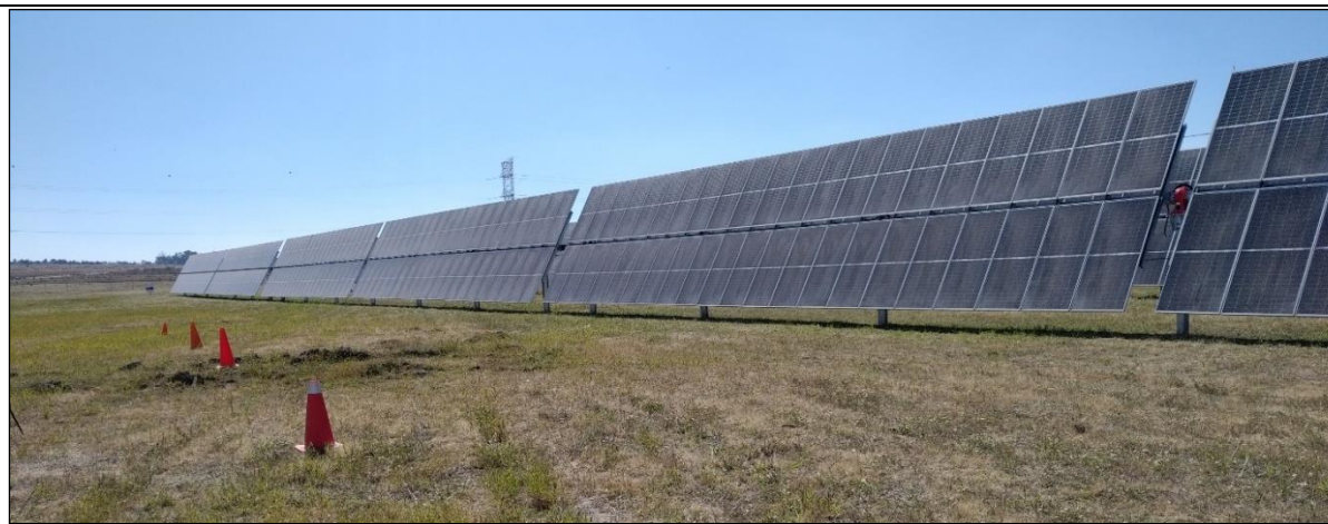
Plate 2-4: Frontal views of the PV arrays mounted on horizontal 1-axis tracker
