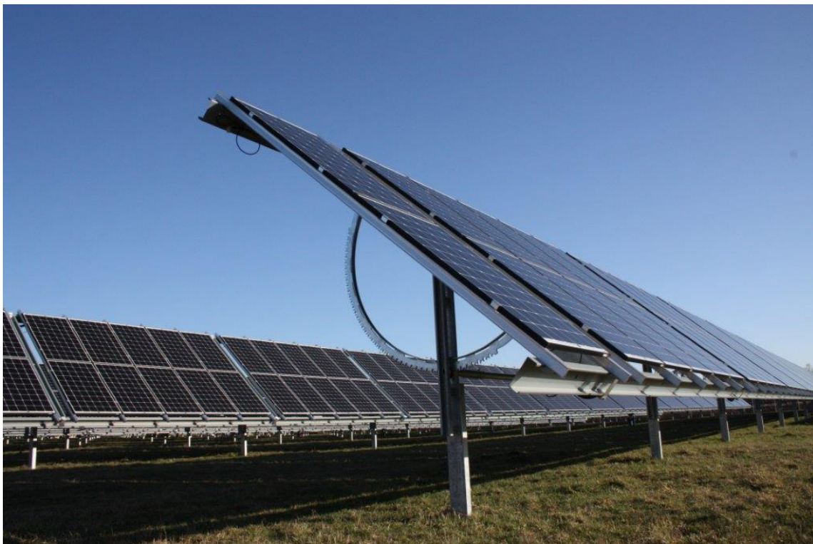
Figure 2: A view of installed single access tracking structures
