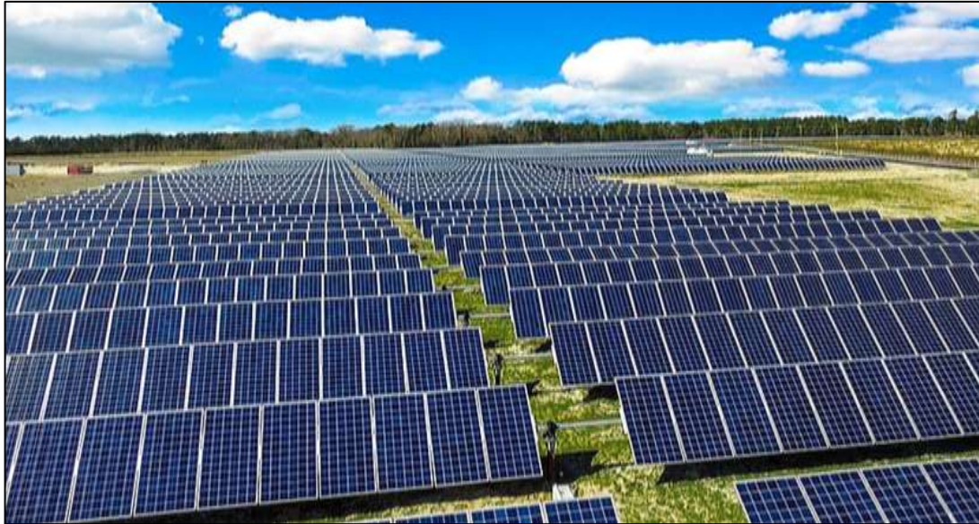
Figure 2.1: Typical example of Solar Power Plant array
