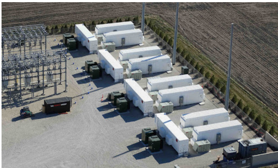
Plate 2-4: A stock image of a similar development with an on-site substation and BESS. Source [ https://reneweconomy.com.au/why-grid-based-battery-storage-is-already-a-no-brainer-in-australia-85967/ ]
