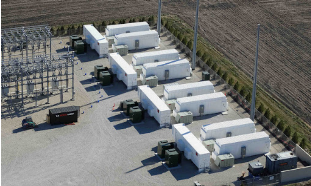
Plate 4-4: A stock image of a similar development with an on-site substation and BESS. Source [ https://reneweconomy.com.au/why-grid-based-battery-storage-is-already-a-no-brainer-in-australia-85967/ ].
