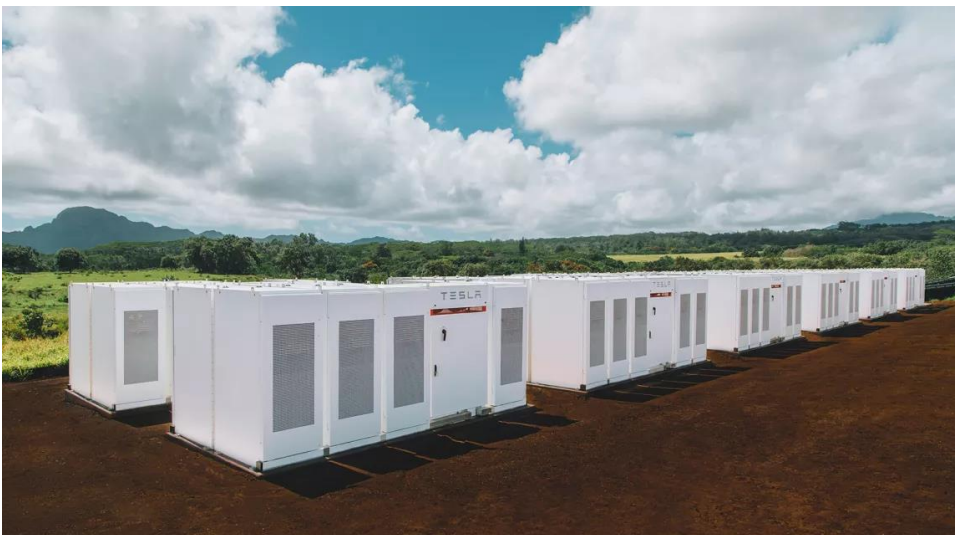
Figure 2.2: Example of battery storage units installed by Tesla (Source: fastcompany.com)
