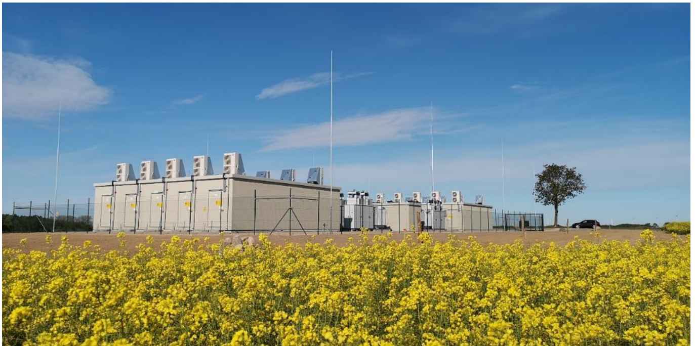
Figure 4.5: Li-Ion BESS implementation for a Renewable Energy facility (Source: Enel Green Power).
