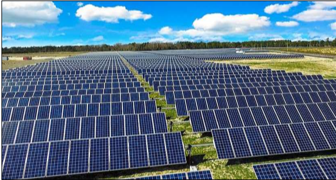
Figure 2.1: Typical example of Solar Power Plant array
