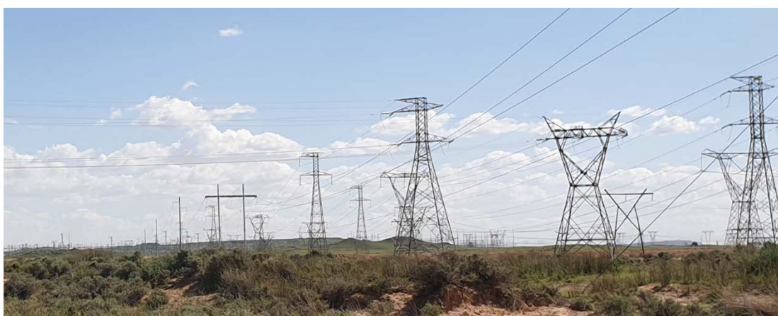
Plate 5-2: Multiple electricity transmission lines exist in the area, converging on the Hydra Main Transmission Substation.
