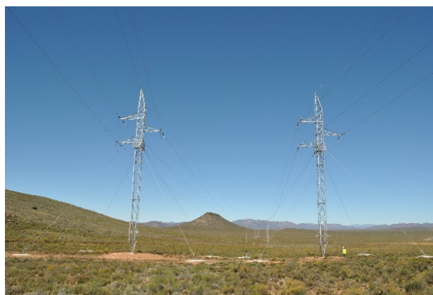
Plate 7-2: Guy line supported steel structures.
