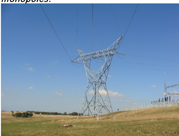
Plate 7-3: Freestanding metal lattice towers.
