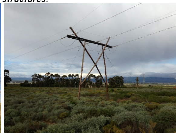
Plate 7-4: Multi-pole structures such as H-towers or K-towers.
