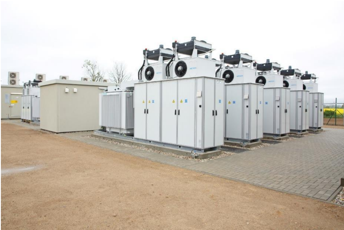
Figure 4.9: Li-Ion BESS containerised modules located within the BESS enclosure footprint (Source: Enel Green Power)
