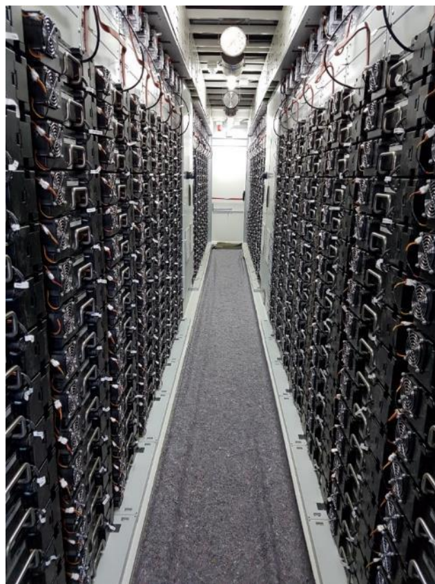
Figure 4.10: Li-Ion BESS internal design and implementation of a container used within a BESS. The image shows a series of sealed battery cell packs within a containerised module (Source: Enel Green Power)
