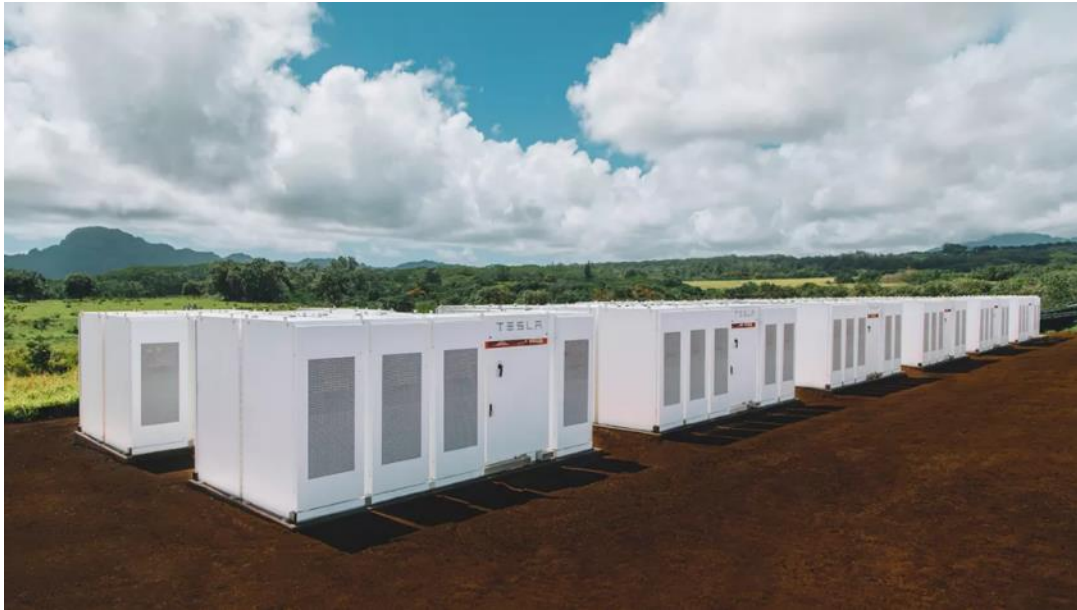
Figure 4.11: Illustration of battery storage units installed by Tesla (Source: fastcompany.com)
