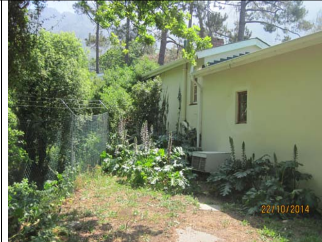
Figure 8: West view of the rear portion of the Fynbos Lodge directly adjacent to the Liesbeck River to the South.
