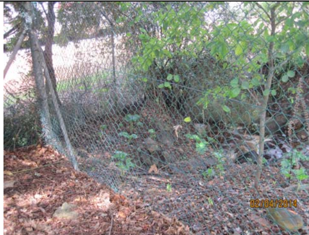
Figure 12: South-east view of Culvert B directing the Liesbeck river beneath Rhodes Drive.
