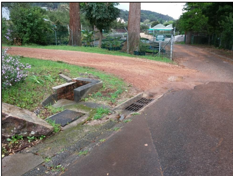
Figure 1: Typical Example of existing stormwater infrastructure.
