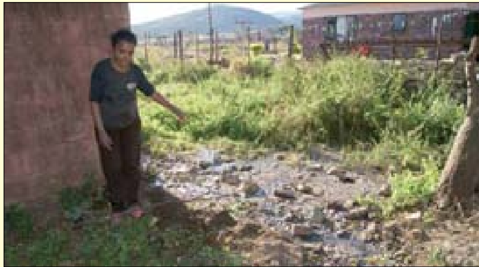
Ms Jowien Williams (47) stands near a pool of sewage at the back of her house at Tshikota in Makhado.
