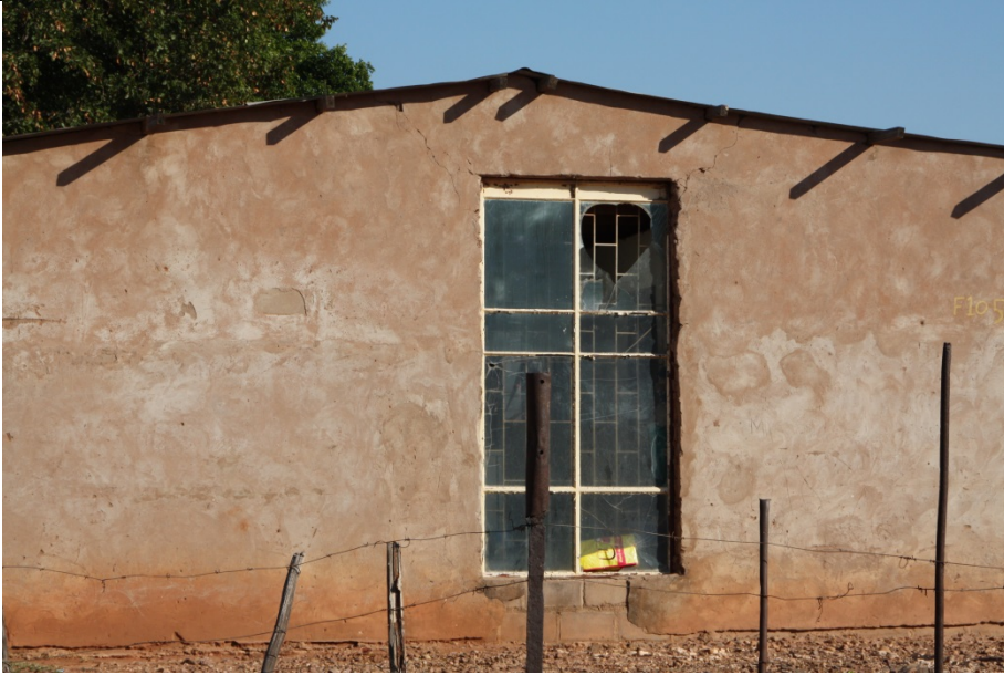
Plastered house with typical damages observed
