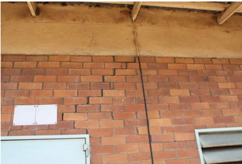
Figure 10: Example of blast induced damage.
