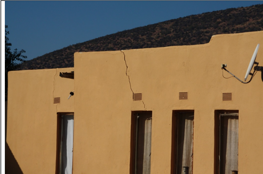
House with very prominent vertical crack
