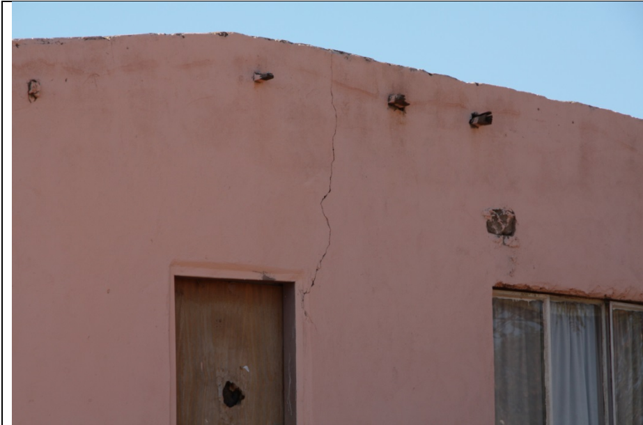
House with very prominent vertical crack
