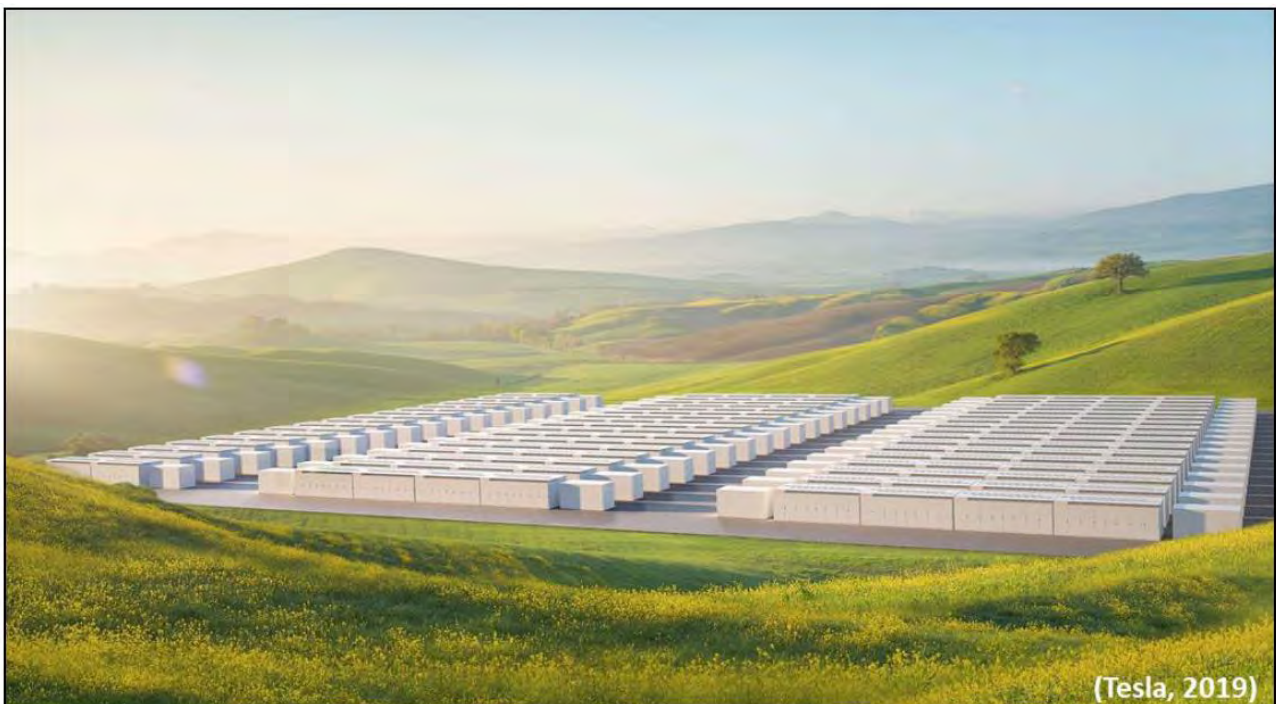
Figure 2-6: Tesla's Megapack Li-ion Battery (Modular System).
