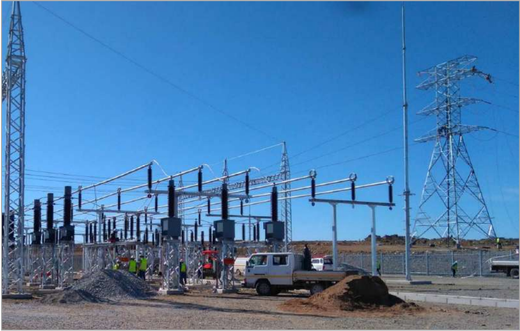
Figure 19: Example of High Voltage Transmission Line Connecting to Substation
