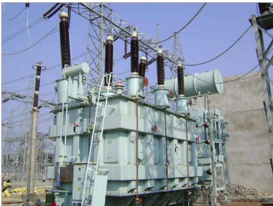
Figure 12: Example of Medium Voltage Transformer (source: https://www.ulaginoli.com/ )
