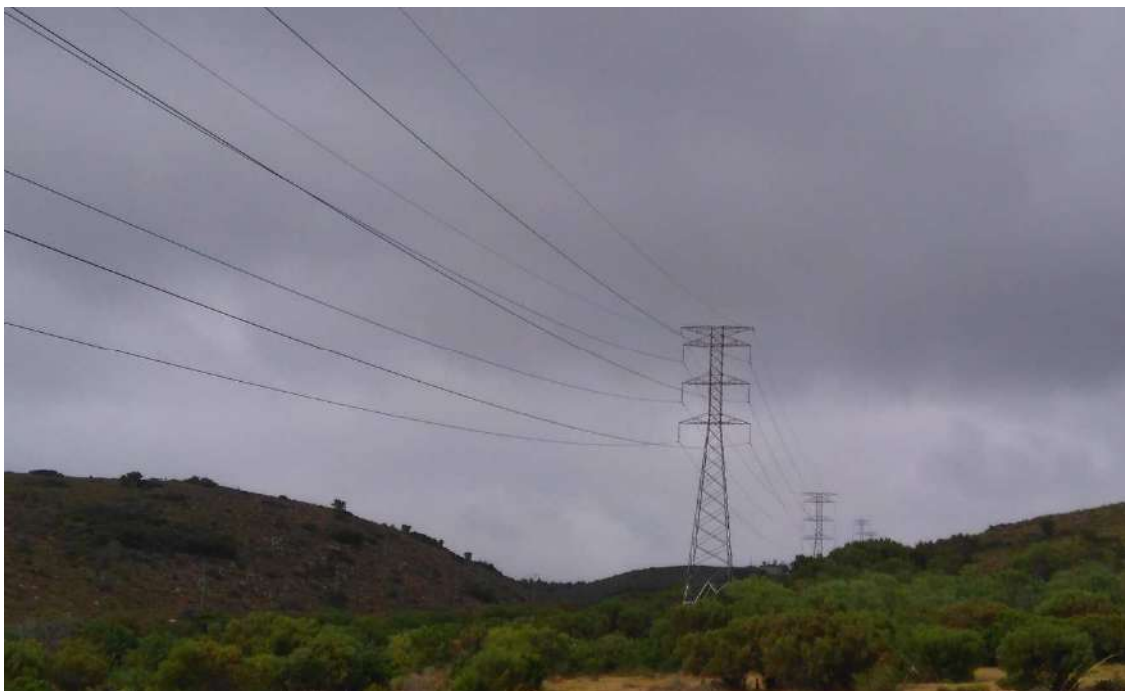
Figure 18: Example of a 132 kV transmission line
