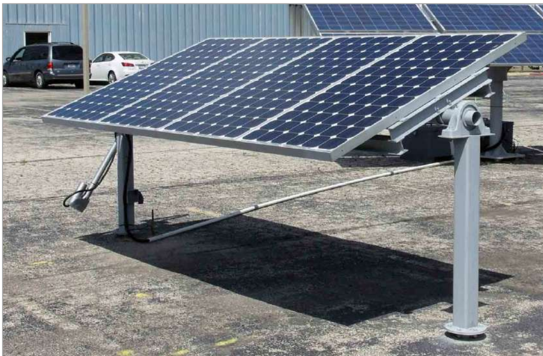
Figure 11: Example of PV Module mounted on Single Axis Tracker (source: Single-ACES – Atlantic Clean Energy Supply – Official Site [ https://atlanticces.com/ ])
