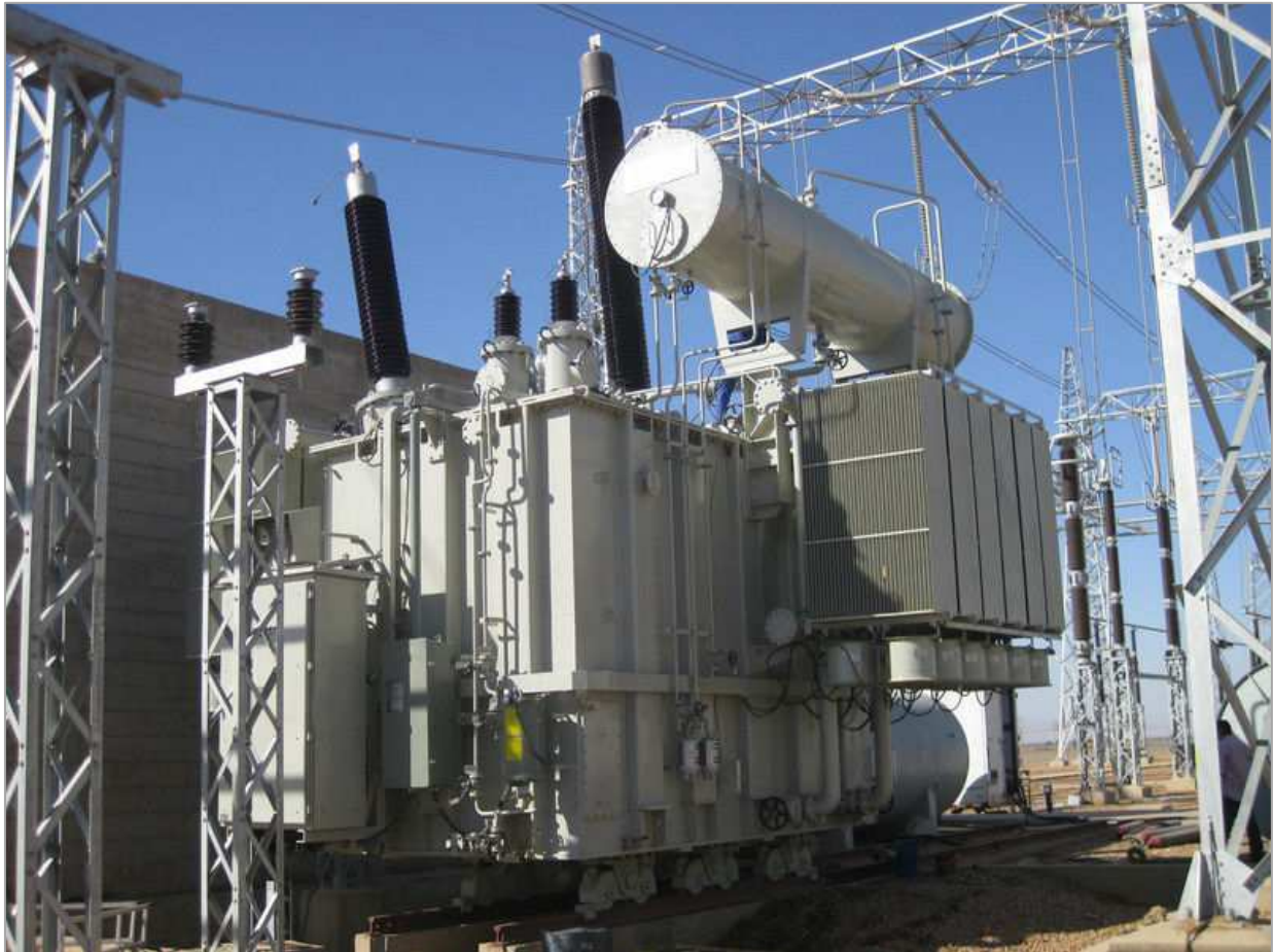
Figure 14: Example of High Voltage Transformers
