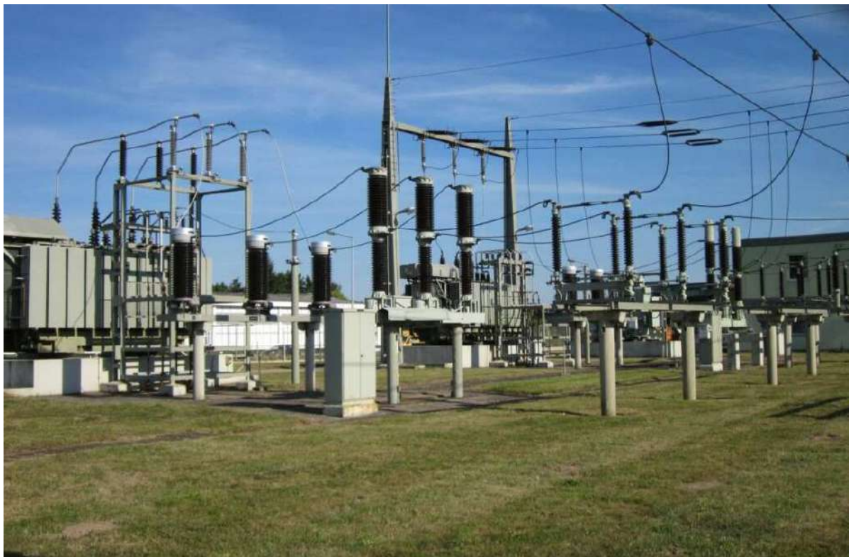
Figure 13: Example of High Voltage Substation
