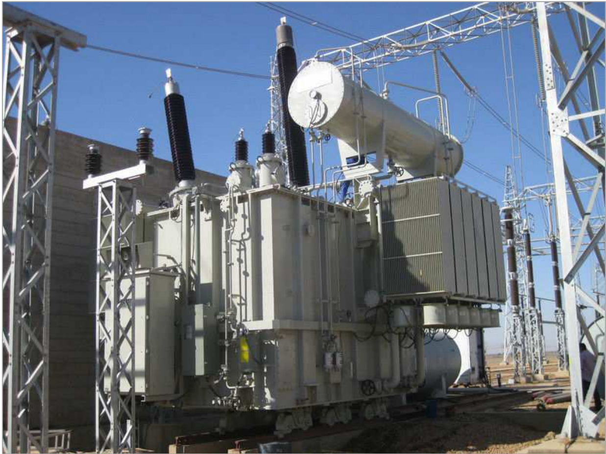
Figure 13: Example of High Voltage Transformers
