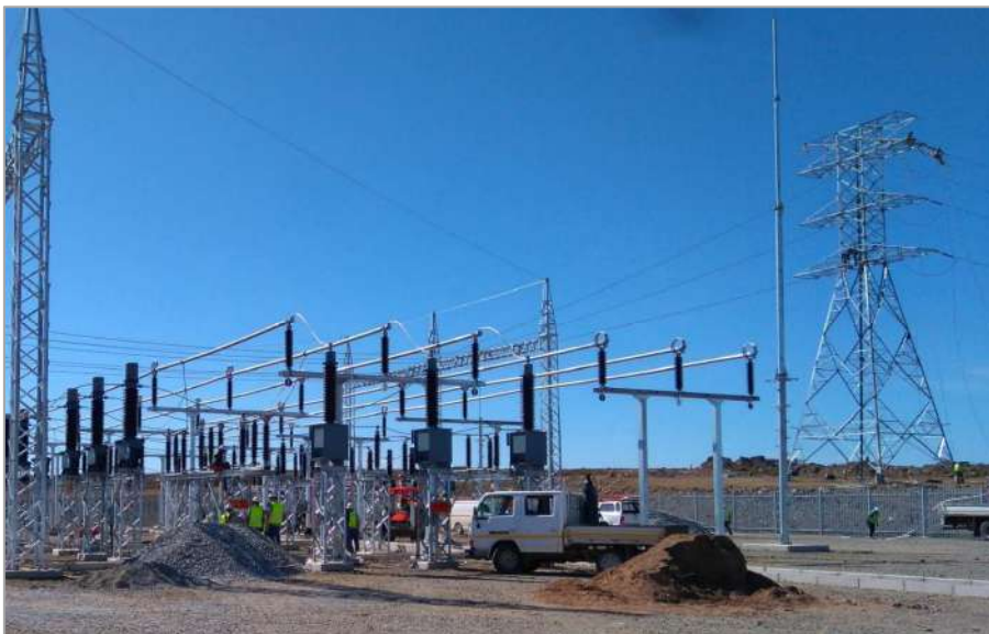
Figure 18: Example of High Voltage Transmission Line Connecting to Substation
