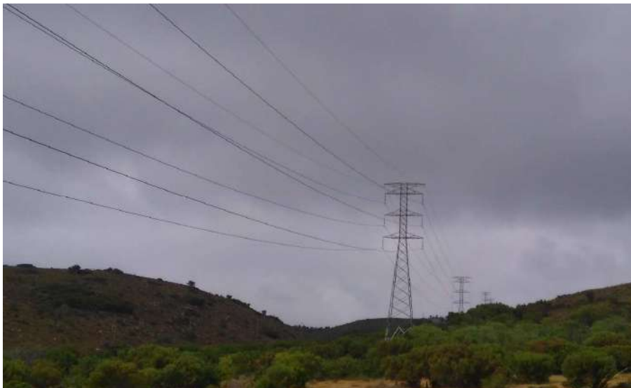
Figure 17: Example of a 132 kV transmission line
