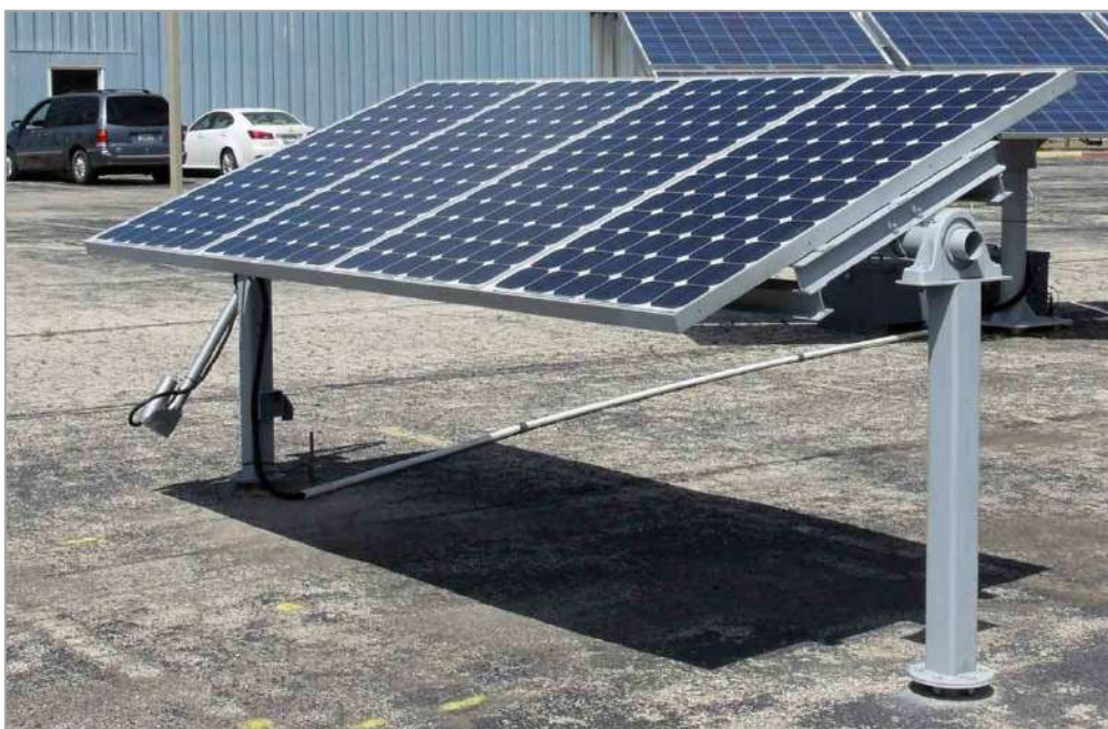
Figure 10: Example of PV Module mounted on Single Axis Tracker
