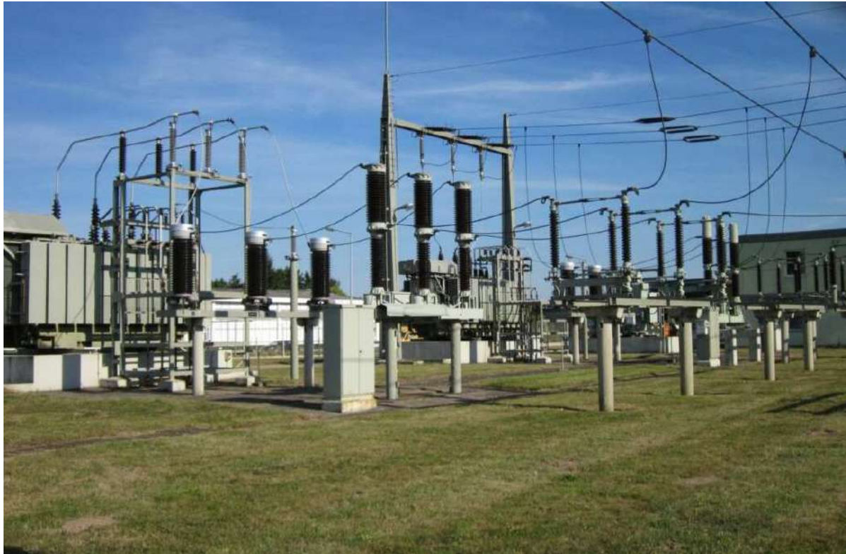
Figure 12: Example of High Voltage Substation
