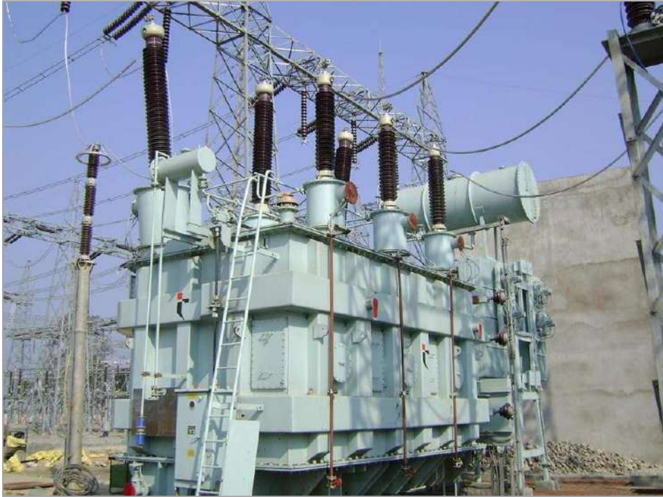
Figure 13: Example of Medium Voltage Transformer
