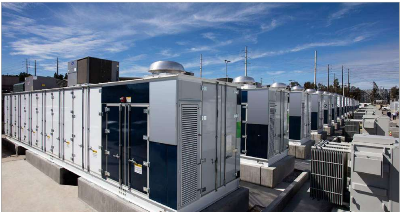
Figure 18: Example of BESS installation ( https://biiworld.com/ )
