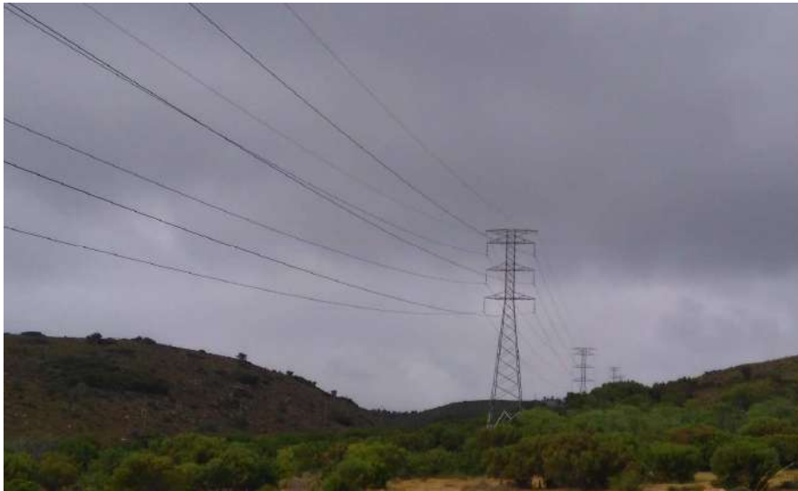
Figure 19: Example of a 132 kV transmission line
