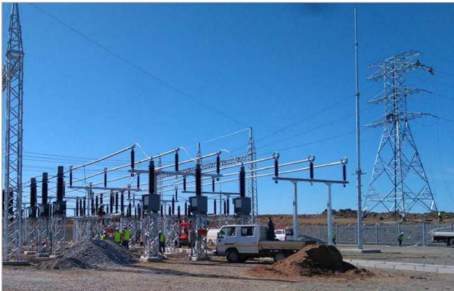
Figure 20: Example of High Voltage Transmission Line Connecting to Substation
