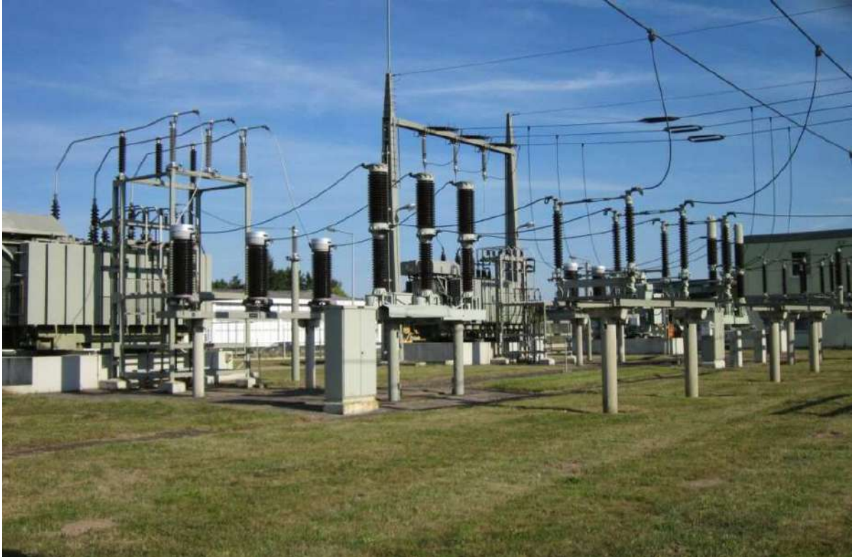
Figure 14: Example of High Voltage Substation
