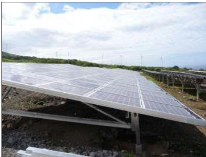
Figure 16: Example of a fixed mounted PV System.
