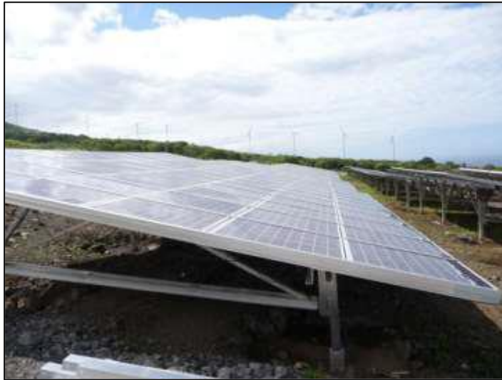
Figure 16: Example of a fixed mounted PV System.
