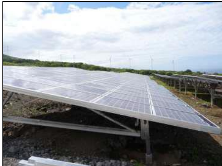
Figure 15: Example of a fixed mounted PV System.
