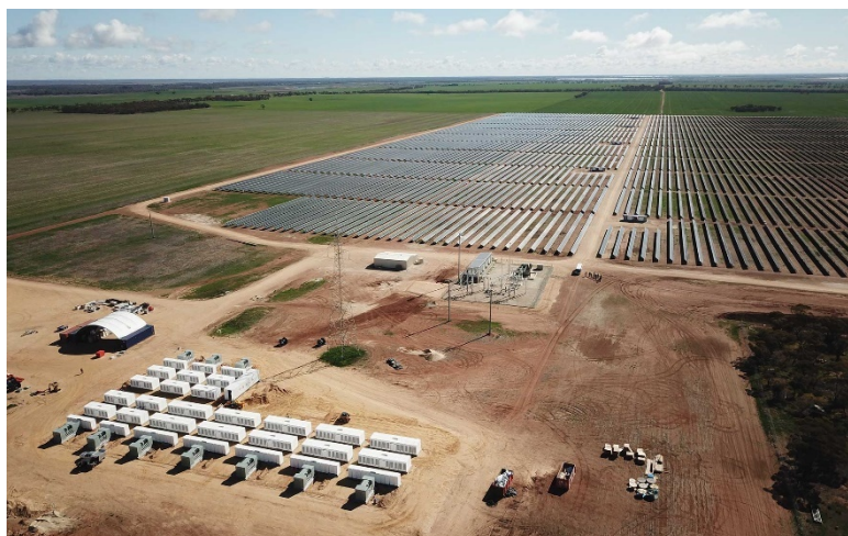
Figure 2.6. Example of PV Technology with Lithium Ion BESS (ARENAWIRE, 2018 3 )
