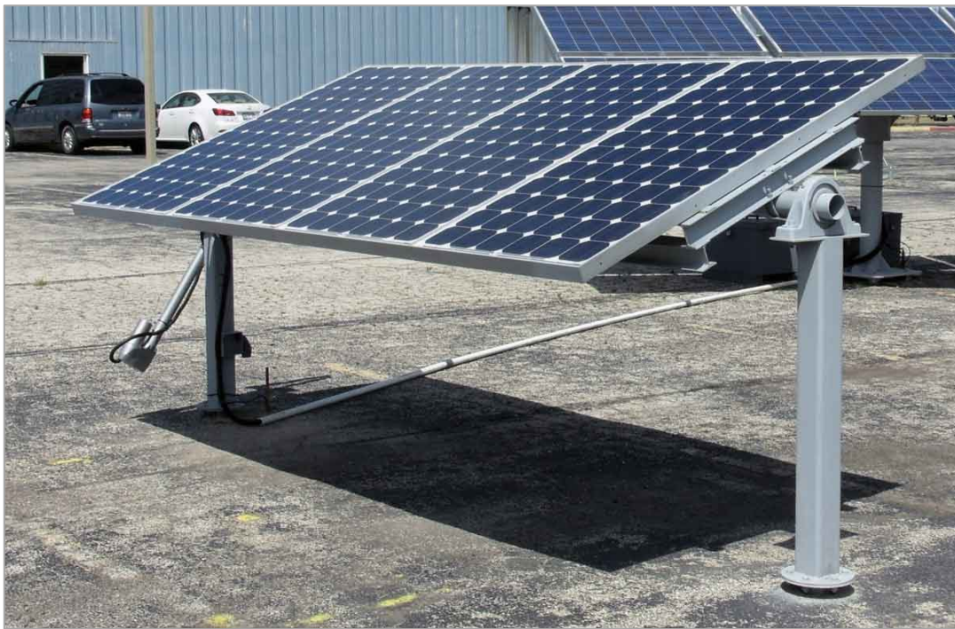
Figure 11 Example of PV Module mounted on Single Axis Tracker
