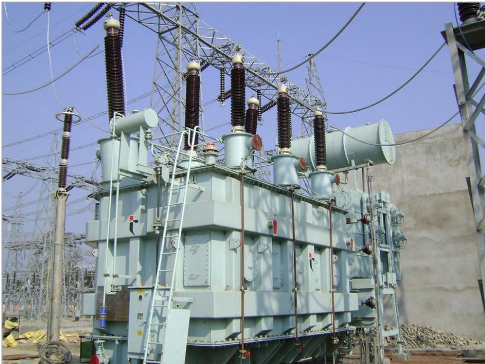
Figure 12: Example of Medium Voltage Transformer (source: https://www.ulaginoli.com/ )
