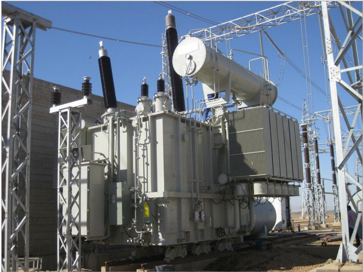
Figure 14: Example of High Voltage Transformers
