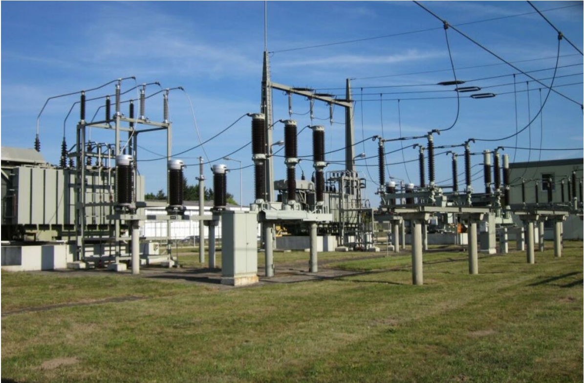
Figure 13: Example of High Voltage Substation
