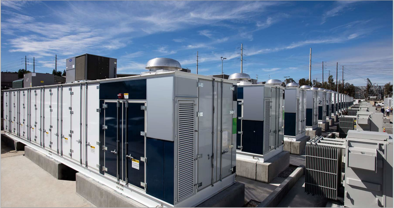
Figure 17: Example of BESS installation ( https://biiworld.com/ )
