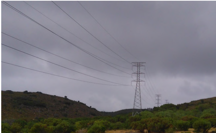
Figure 18: Example of a 132 kV transmission line
