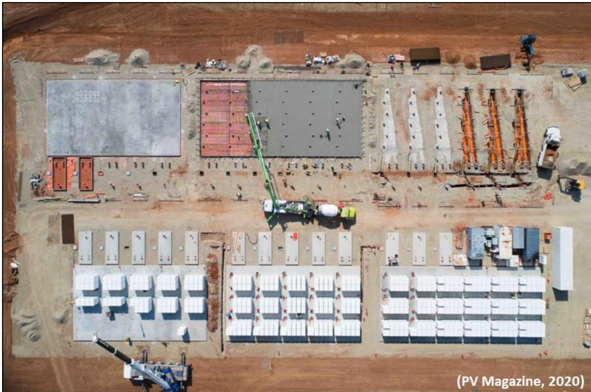
Figure 7: Installation of the 100 MW/129 MWh Li-ion battery at the Hornsdale wind farm
