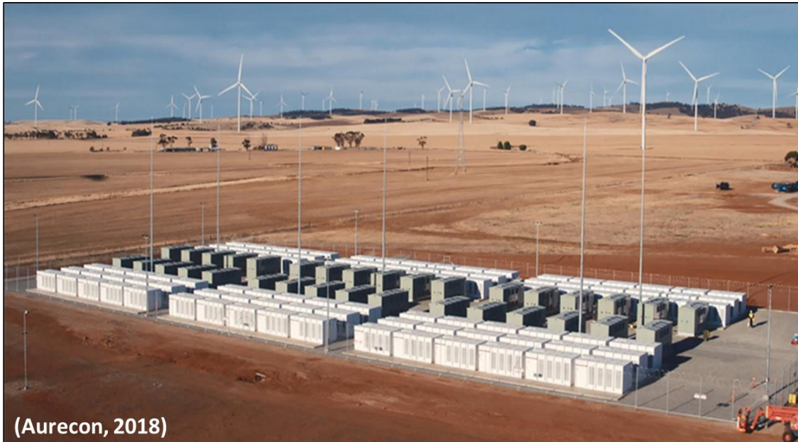
Figure 6: Example of a 100MW/129MWh Lithium-ion battery on the Hornsdale wind farm in Australia.
