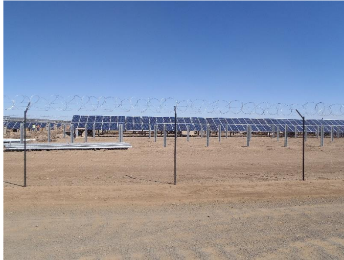
Figure A.7. Example of PV Technology (DEFF, 2019)
