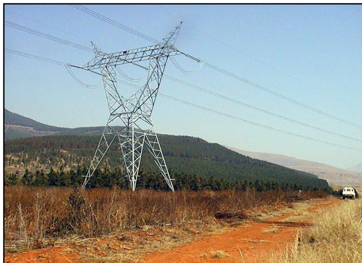
Figure 3: Self-Supporting Strain Tower
