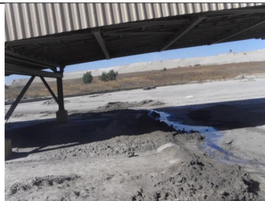
The existing ash dump in the horizon of the photo. A close-up view of the area underneath the conveyor system with a stormwater runoff carrying ash-laden stormwater
