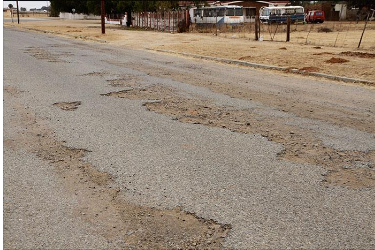
Photo 11: Poor road surface
