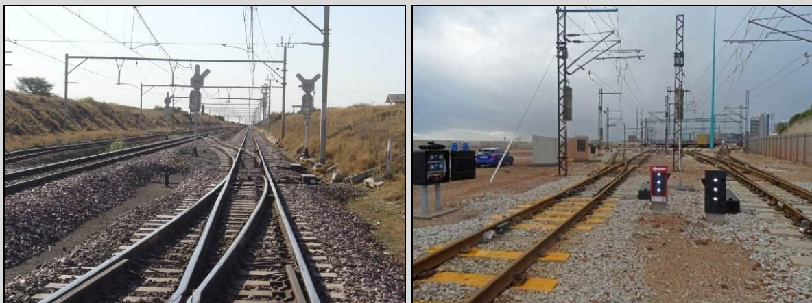
Figure 1.4: An example of a railway perway (left) and typical railway signalling (right).
