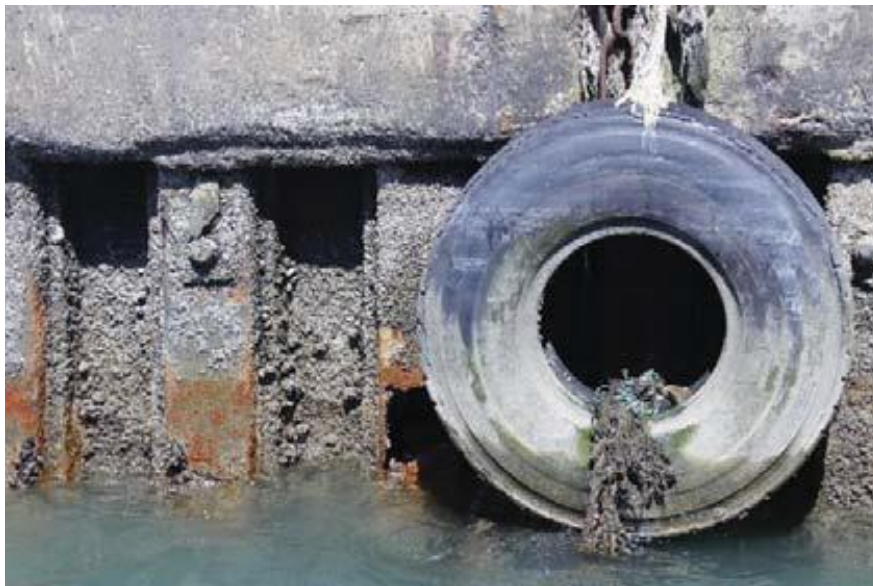
Figure 2: Close-up image indicating the extent of the sheet pile corrosion
