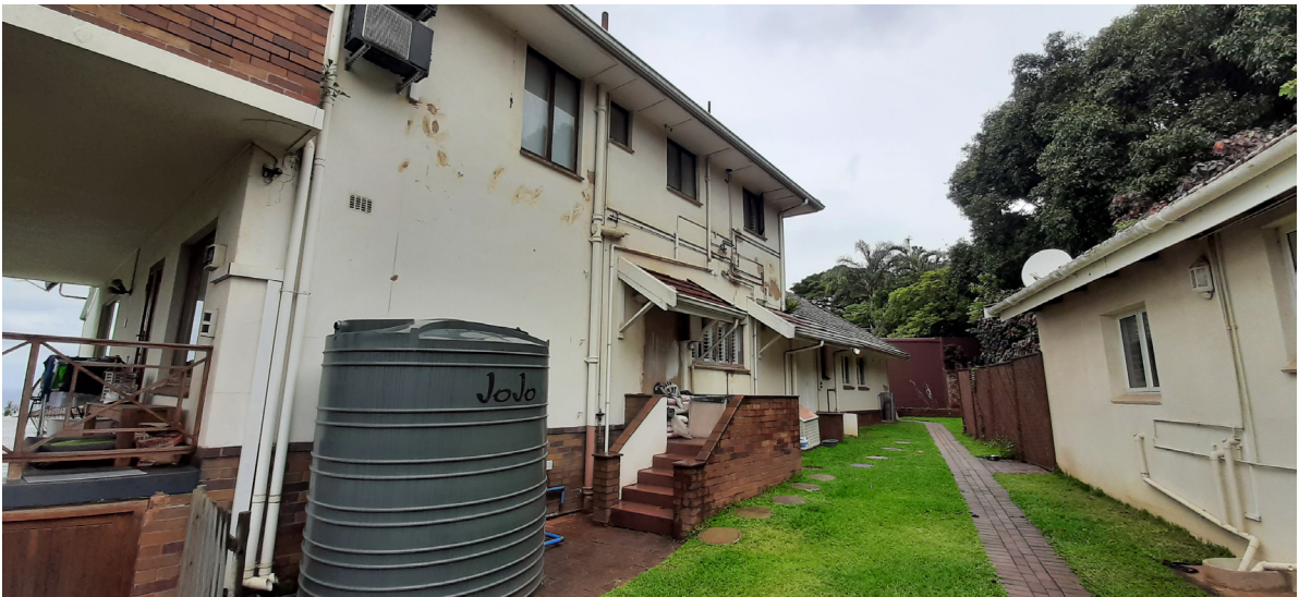
View 14: Rear view (west facade) of the house, with an ancillary unit to the right. Ex dwelling to receive new paintwork as general upkeep.
