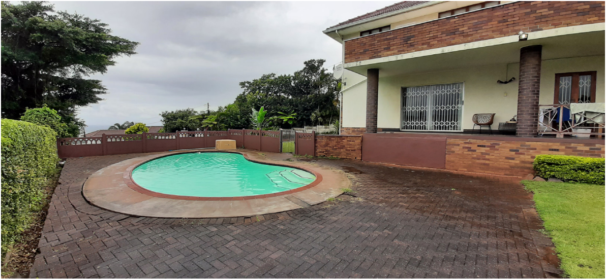
View 13: View looking from the north lawn towards the east / pool, and living spaces facade (right). Exposed brickwork (balcony & columns) to be plastered and painted, to fit in with the new colour scheme of the house.
