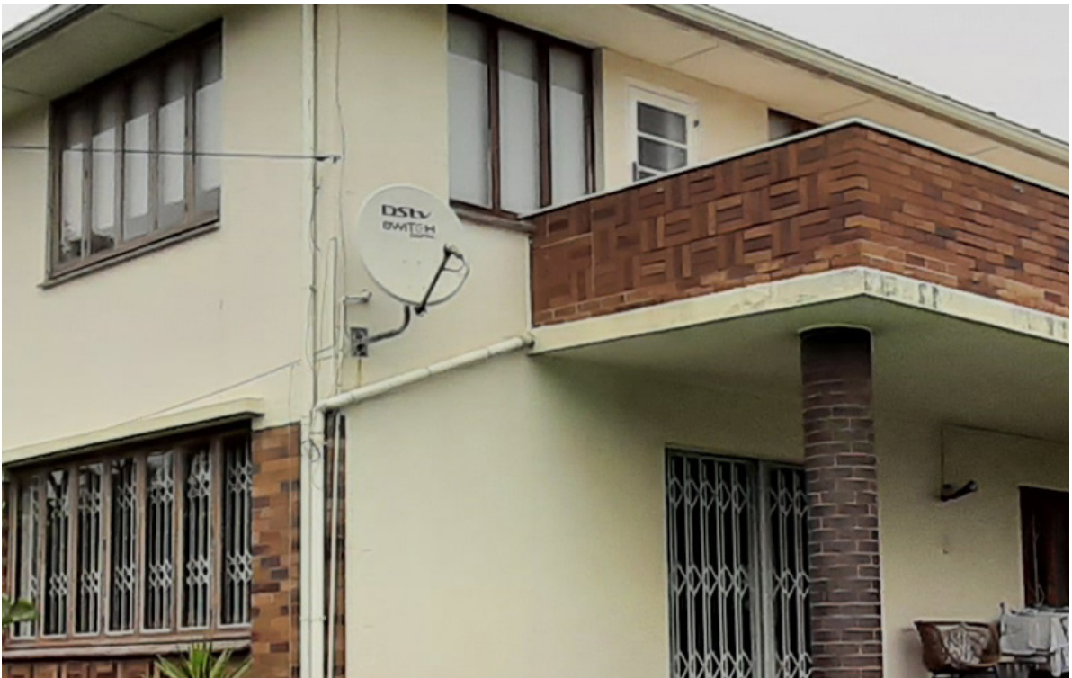
View 28: Existing Window/Door frames to be painted to one uniform colour. Colour as per plans. This is due to them currently having different shades, having been installed at different timelines.
