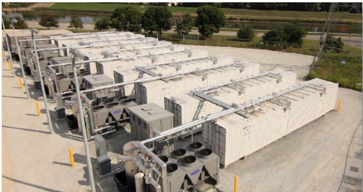
Figure 2.8: Typical layout of a BESS (Source: South Africa Mainstream Renewable Power Developments (Pty) Ltd).
