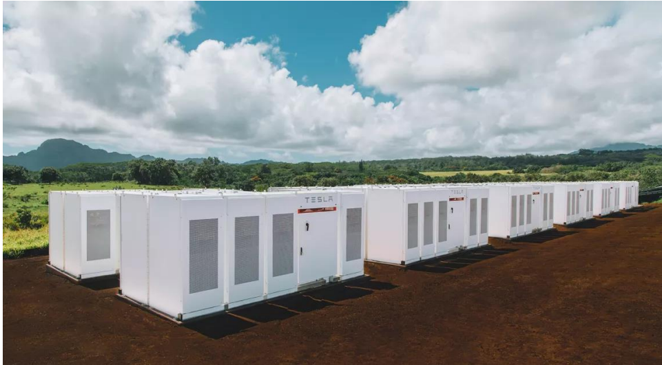
Figure 2.6: Example of battery storage units installed by Tesla (Source: fastcompany.com)
