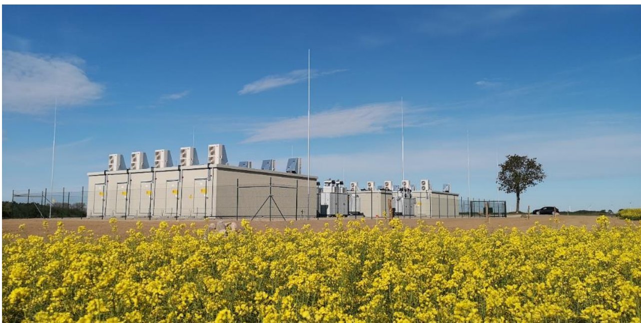
Figure 2.3: Li-Ion BESS implementation for a Renewable Energy facility (Source: Enel Green Power).
