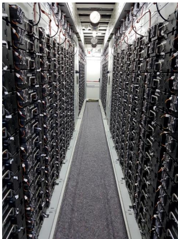
Figure 2.5: Li-Ion BESS internal design and implementation of a container used within a BESS. The image shows a series of sealed battery cell packs within a containerised module (Source: Enel Green Power).
