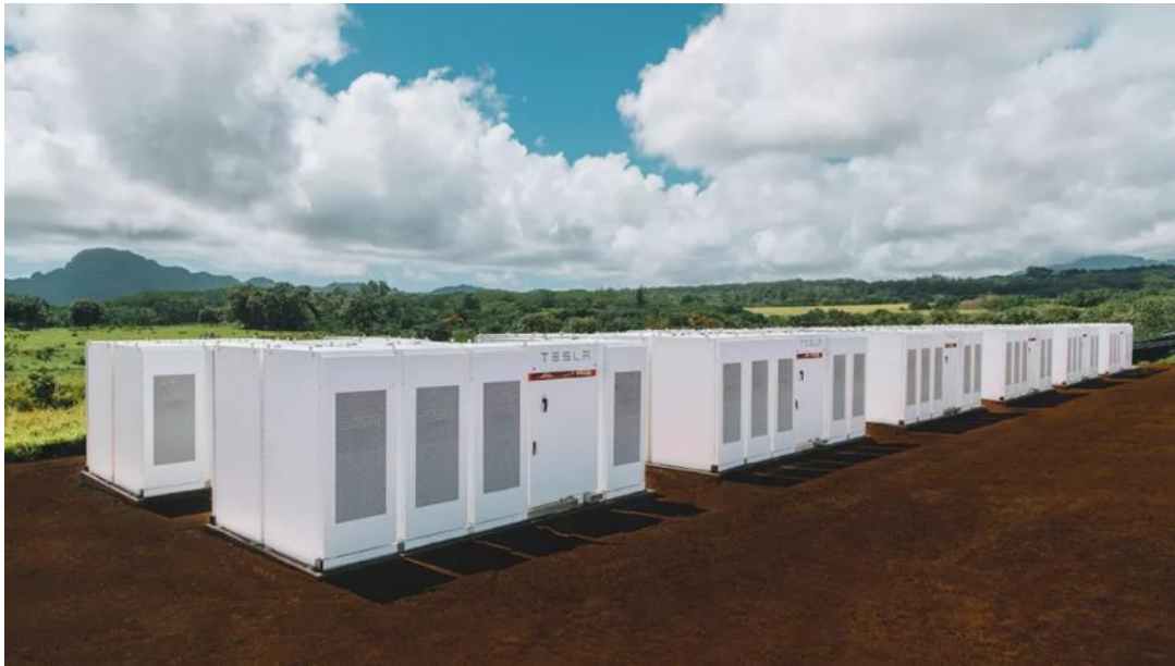
Figure 2.6: Illustration of Lithium-ion battery storage units installed by Tesla (Source: fastcompany.com).
