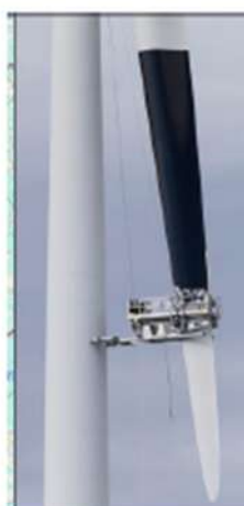
Figure 1: The single black-blade in the process of being painted in situ, at the Smøla Wind Farm. Painting white blades black after they are erected is more expensive than producing them at source.
