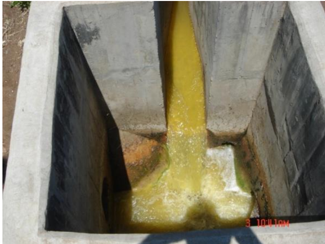
Photo 5: Flow at Dzanani sewage treatment works
