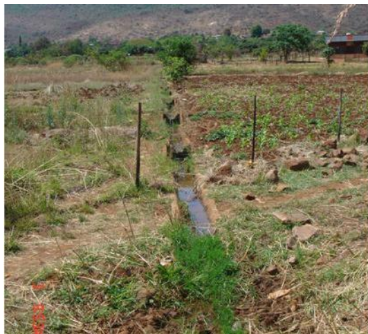
Photo 6: Poorly maintained canals
