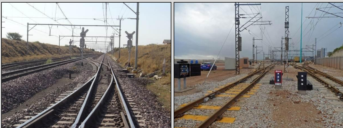
Figure 1.4: An example of a railway perway (left) and typical railway signalling (right).
