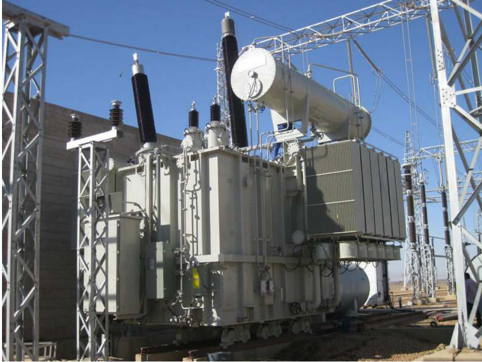
Figure 13: Example of High Voltage Transformers
