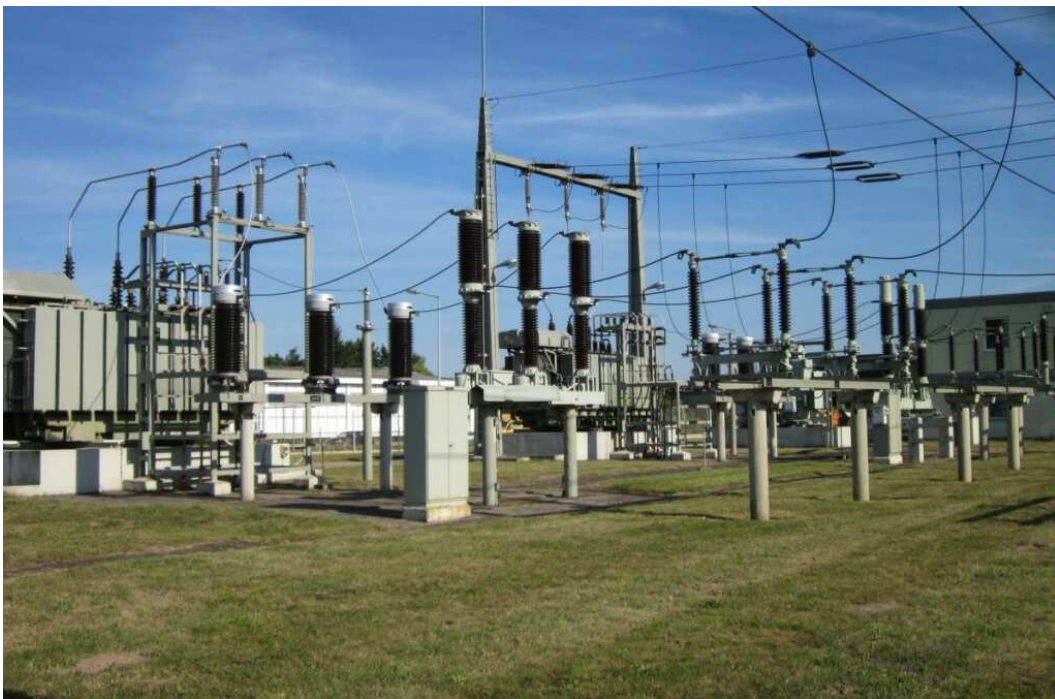
Figure 12: Example of High Voltage Substation
