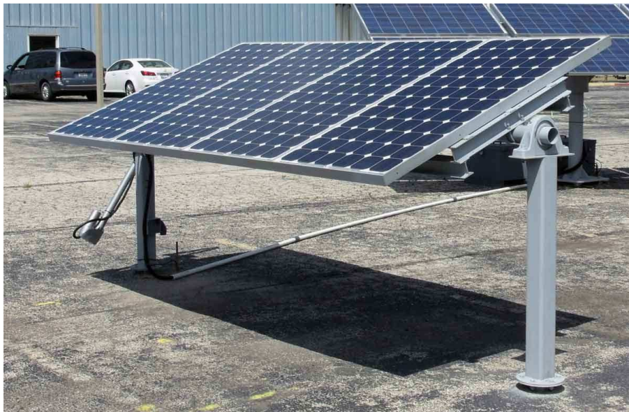
Figure 10: Example of PV Module mounted on Single Axis Tracker (source: Single-ACES – Atlantic Clean Energy Supply – Official Site [ https://atlanticces.com/ ])
