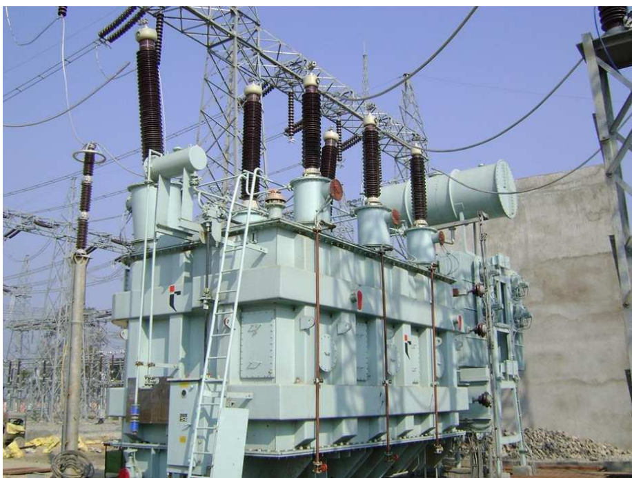
Figure 11: Example of Medium Voltage Transformer (source: https://www.ulaginoli.com/ )
