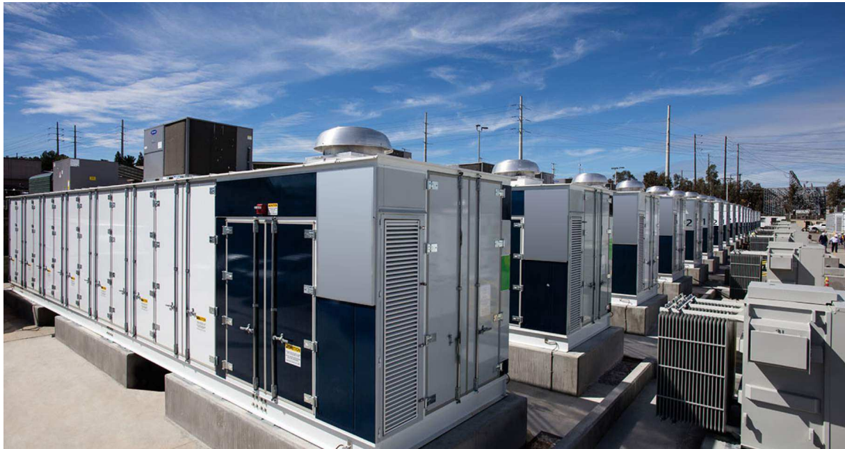
Figure 16: Example of BESS installation ( https://biiworld.com/ )
