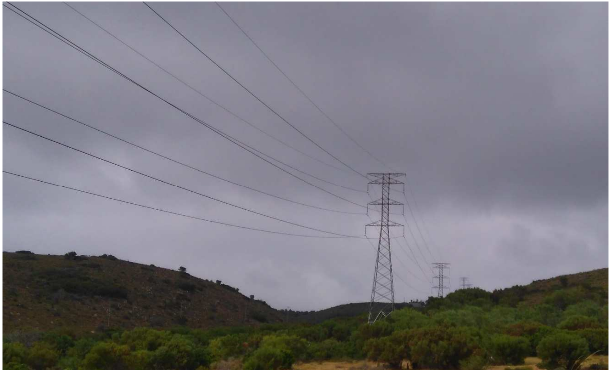
Figure 17: Example of a 132 kV transmission line
