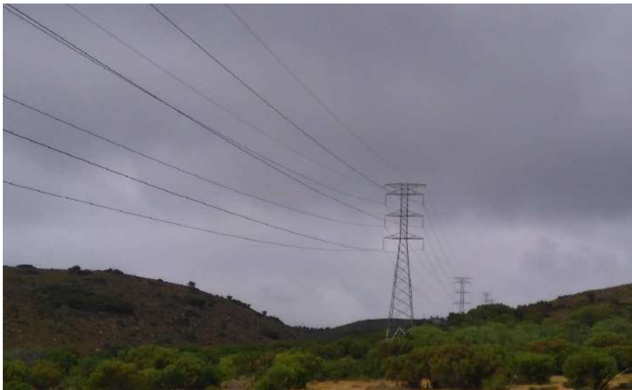
Figure 19: Example of a 132 kV transmission line
