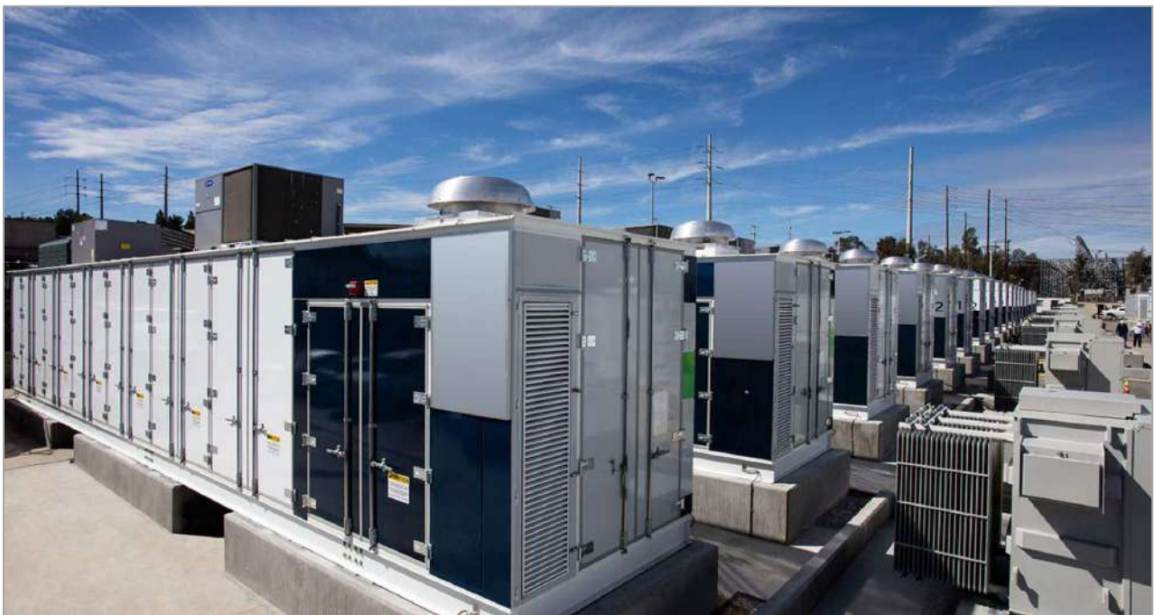
Figure 18: Example of BESS installation ( https://biiworld.com/ )
