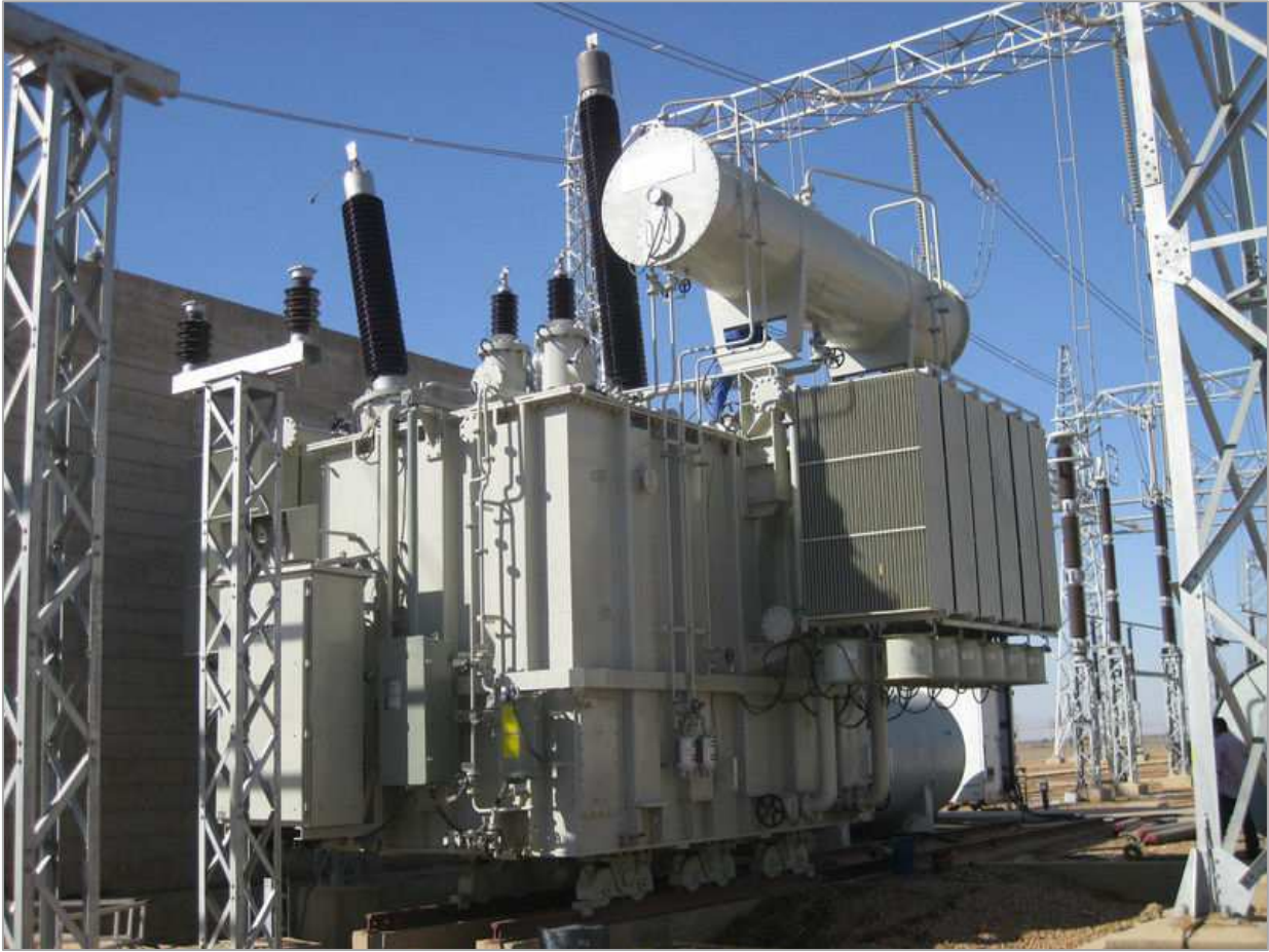
Figure 15: Example of High Voltage Transformers
