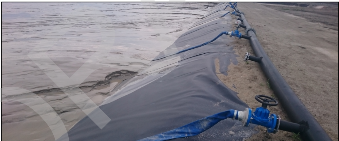
Figure 6-4: Multiple Spigot Discharge (Maseve Platinum Mine, South Africa)
