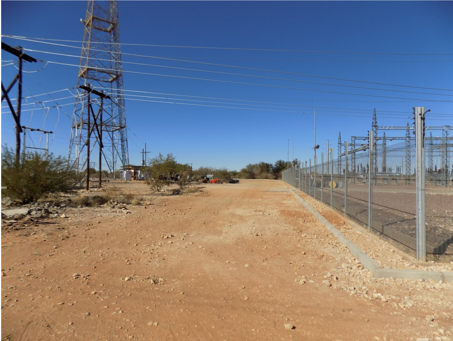
Figure 5 West boundary of Cuprum substation viewed from the south west corner of the substation ( 29^{\circ}57'33.65''\text{S} ; 22^{\circ}17'57.98''\text{E} )
