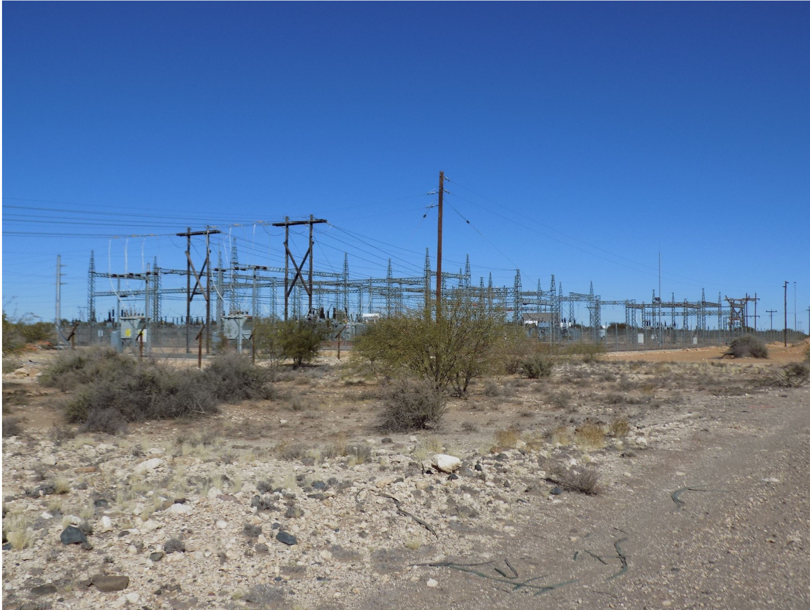
Figure 1 Cuprum substation viewed from the north west corner of the study area ( 29°57'29.47"S; 22°18'1.95"E)
