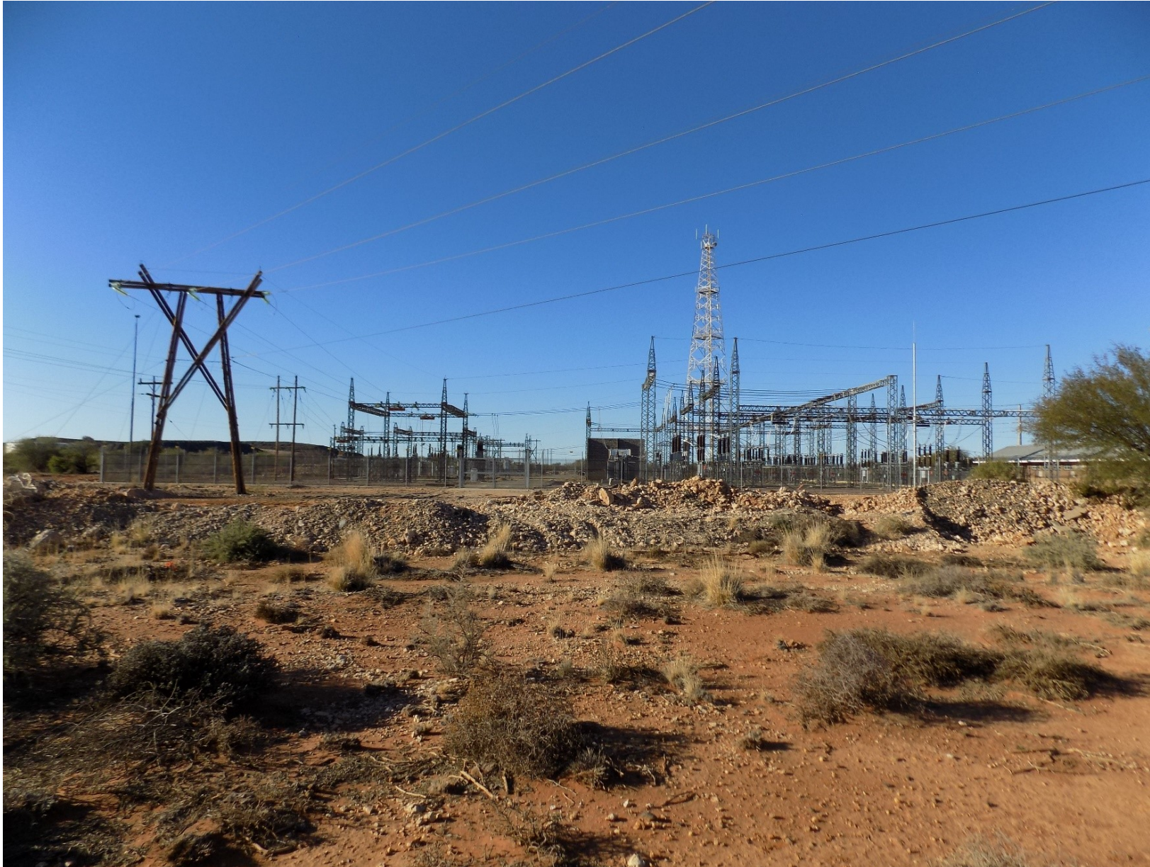
Figure 9 South of the Cuprum substation and proposed location of the substation extension and road extension ( 29°57'36.01"S; 22°17'58.12"E)
