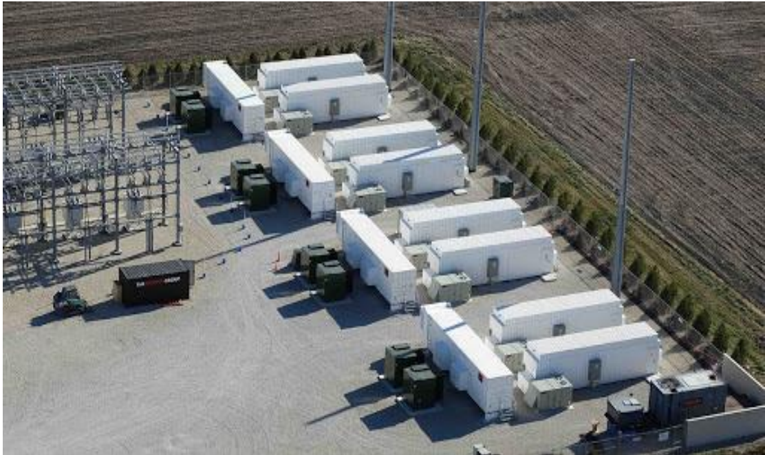
Plate 2-3: A stock image of a similar development with an on-site substation and BESS. Source [ https://reneweconomy.com.au/why-grid-based-battery-storage-is-already-a-no-brainer-in-australia-85967/ ]
