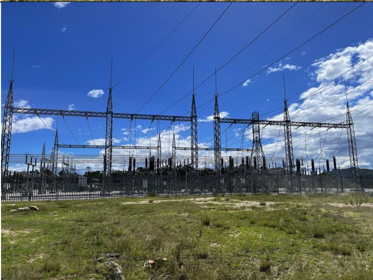
The Eskom (Humansdorp) Substation located on the southwest corner of the study site.
