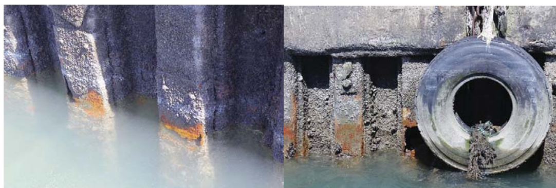
Figure 1-2: Extent of sheet pile corrosion
