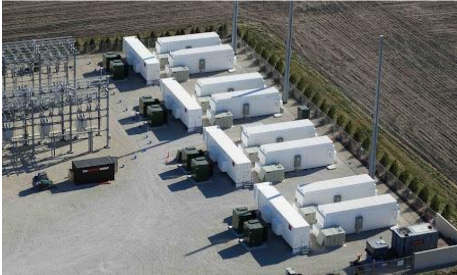
Plate 2-4: A stock image of a similar development with an on-site substation and BESS. Source [ https://reneweconomy.com.au/why-grid-based-battery-storage-is-already-a-no-brainer-in-australia-85967/ ]
