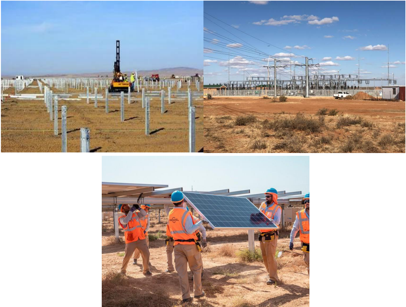
Figure 2-6: Photographs depicting the construction phase of a solar farm similar to Red Sands Solar East SEF. Source:
