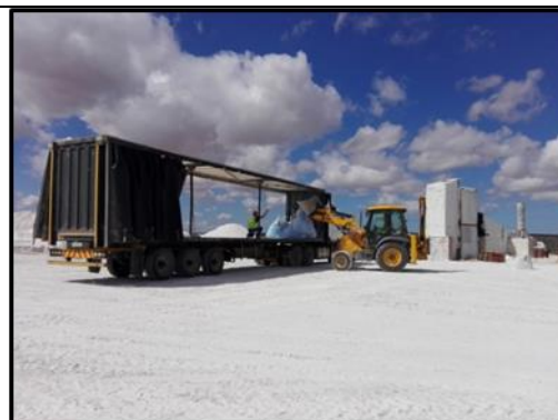
Photograph 3: View of the Backhoe Actor loading a bag of kaolin onto the truck for hauling off site.
