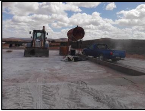
Photograph 4: View of the bunded area for the diesel bowser and parking area for the Front-End Loader.
