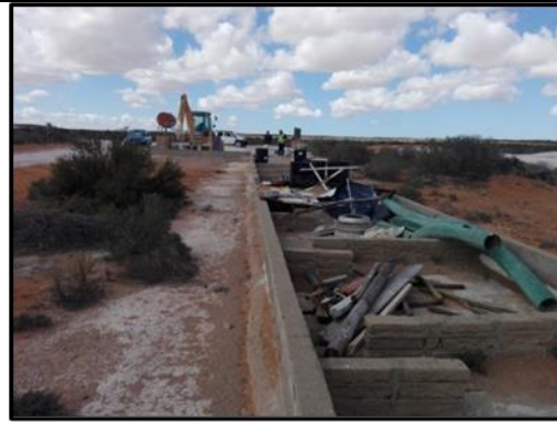
Photograph 5: View of the materials storage area, neatly separated and bunded. Soil farm areas for spillages of hazardous substances are located closer to the diesel bowser bunded area.
