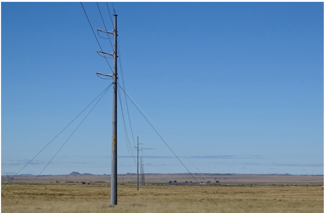
Figure 2: Example of monopole where powerlines cross the R48 Route north of De Aar
