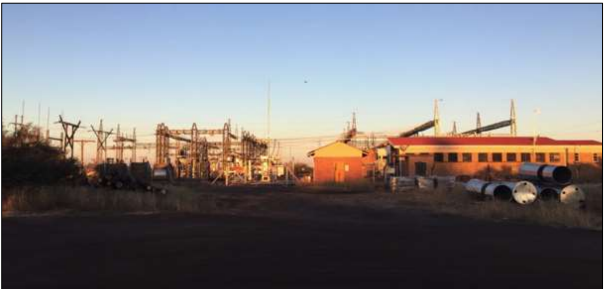
Figure 7: View west from Photo 6 of the existing Hotazel Substation to which the proposed power line would be routed.
