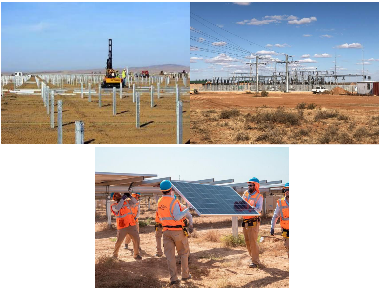
Figure 2-5: Photographs depicting the construction phase of a solar farm similar to De Rust PV1 SEF. Source:
