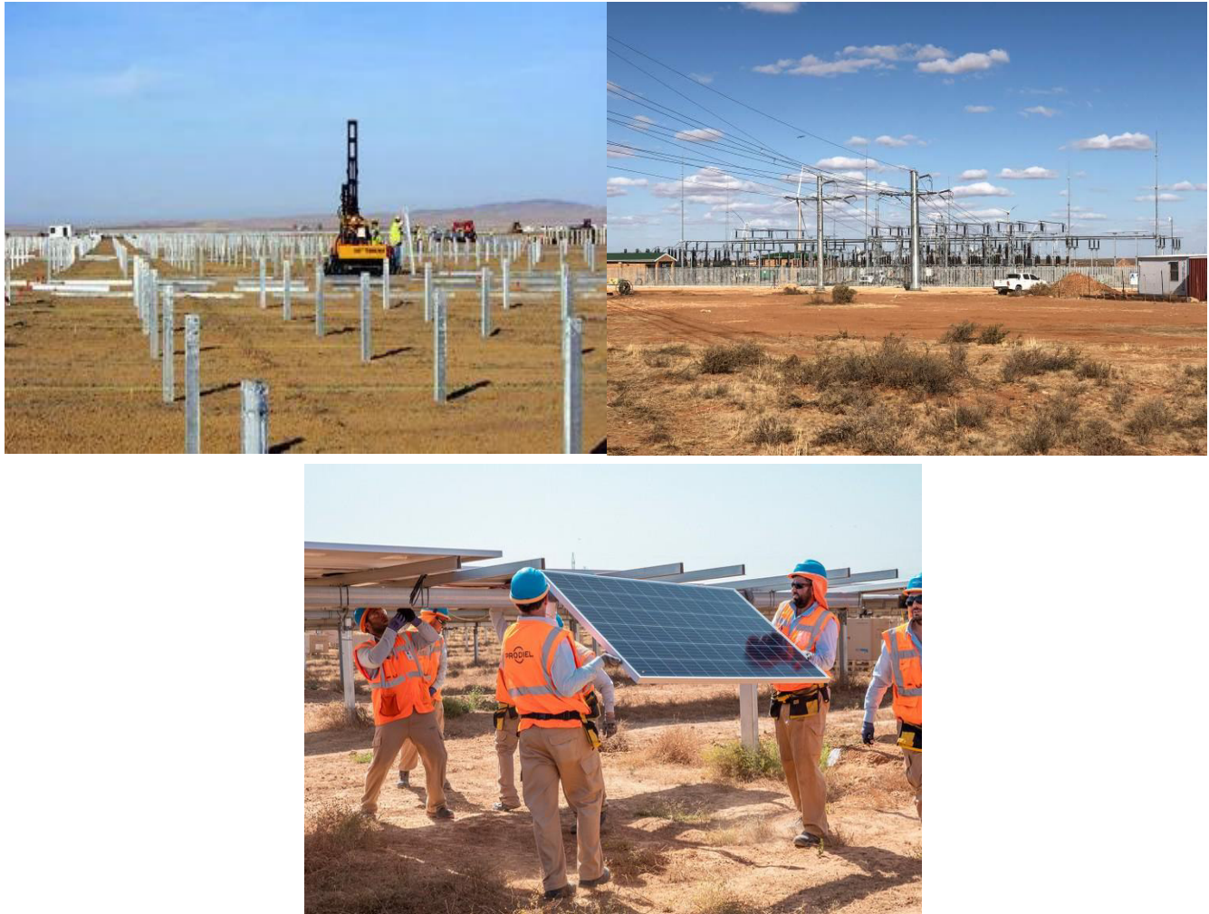
Figure 2-5: Photographs depicting the construction phase of a solar farm similar to De Rust PV2 SEF. Source:
